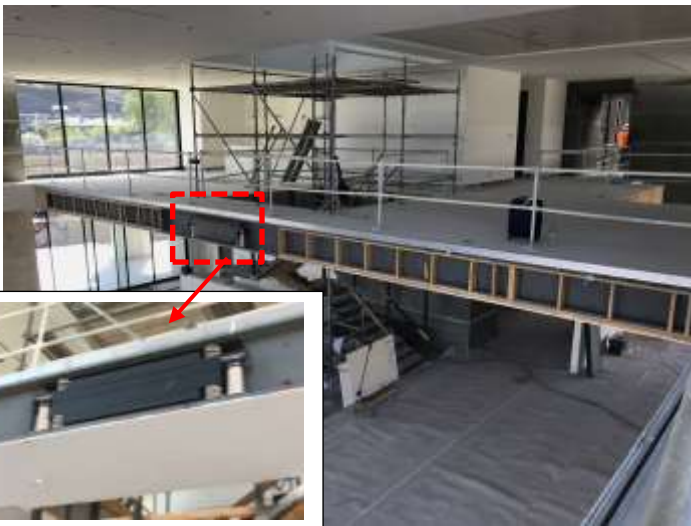
Figure 1 The 60 ft span balcony with the TMD
